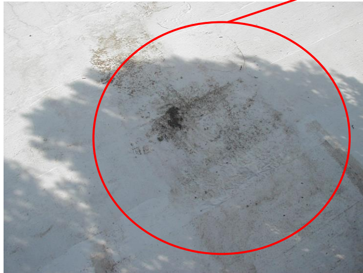
RC.1 Surface Coating Needed
